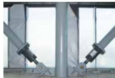
The dampers are installed at the bottom end of the cross braces. They have a length of 750 mm.
