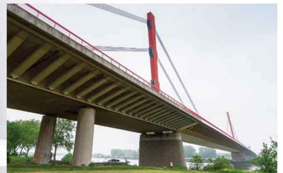
The two steel pylons of the cable-stayed bridge have a height of 66.7 m and are located in the center axis of the bridge. On each side, three harp-shaped cable groups are anchored in the pylons.
