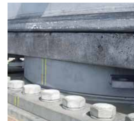
The bearings underneath the Bogibeel Bridge transmit a load of 2,800 t in the smallest of spaces.
